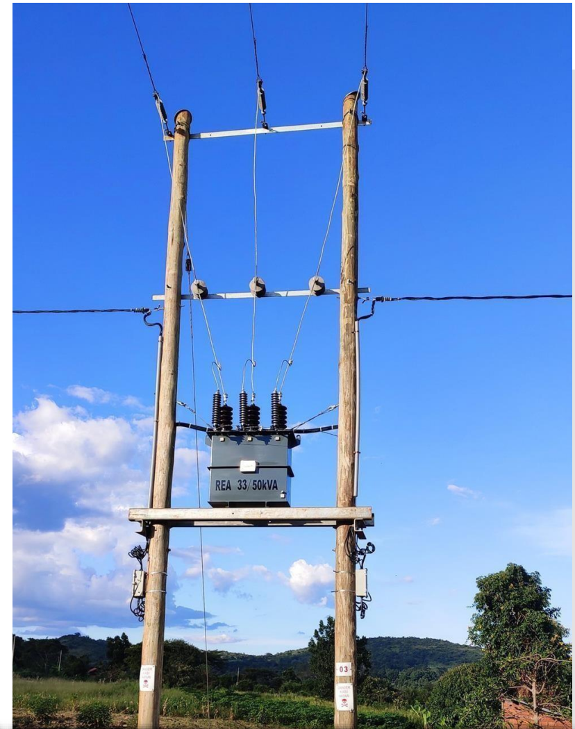
Completed Installation & Commissioning of Transformer 33/50 kVA Scheme 44, Lot 5 Project Masodde Kyankwanzi District.
