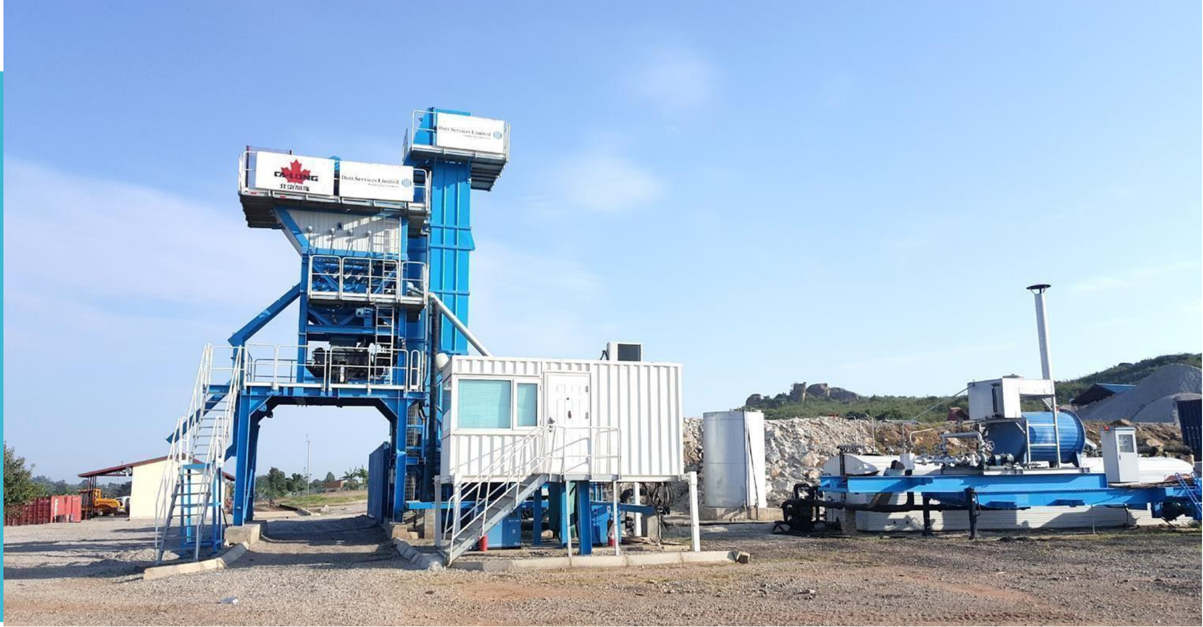
ASPHALT PLANT IN MBALE QUARRY, UGANDA
