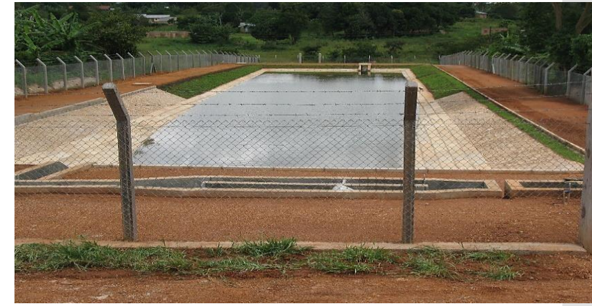
Constructed Hoima Sewerage System
