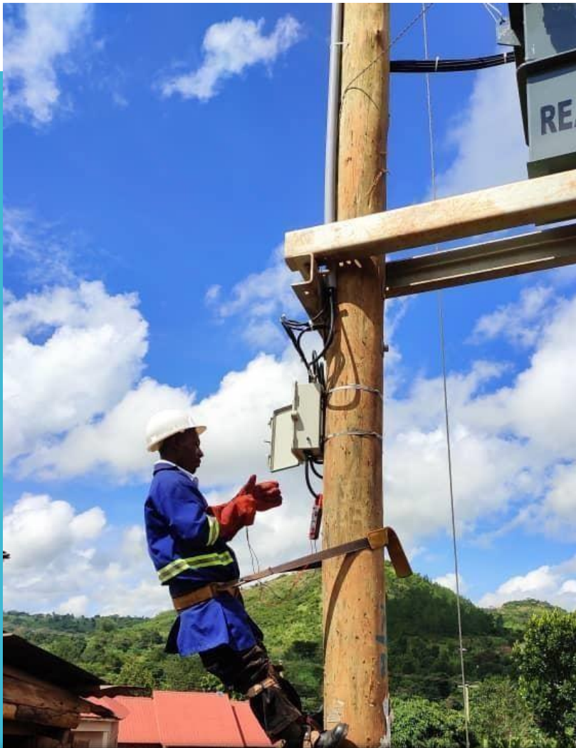
Test at Commissioning of 33KV Transmission line project -Scheme 36, Lot 5 Project - REA
