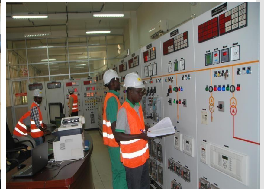
COMPLETED INSTALLATION OF PLC & CONTROL ROOM IN POWERHOUSE - BUSERUKA, HOIMA, UGANDA
